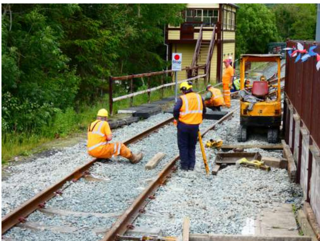
Track Engineer, Dave Shaw (kneeling) checks alignment and radius after the track has been slewed over Photo: DT
