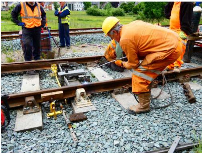
Paul Whitton heating up the rail to aid bending the curve Photo : DT
