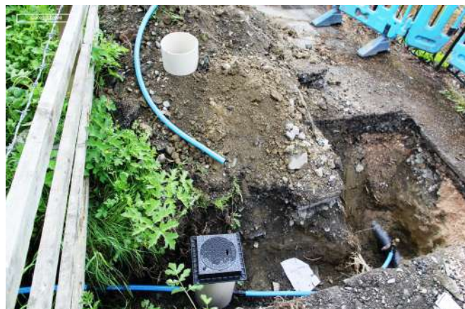
The long awaited mains water connection complete with stop valve Photo : PN
