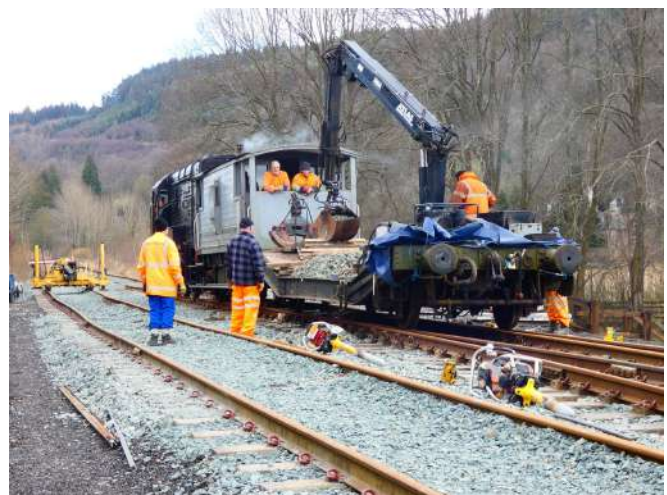
Lowmac/Atlas Crane helps to redistribute some of the ballast Kango tampers next to track Photo : MW
