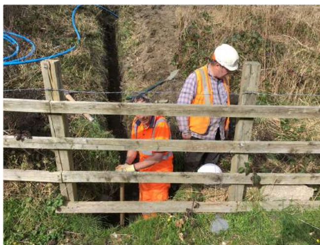
Hoping that the correct depth has been reached for the blue water pipe and that the work is now acceptable?
