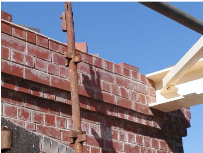
Top course of bricks now complete on east end of building Photo : PR
