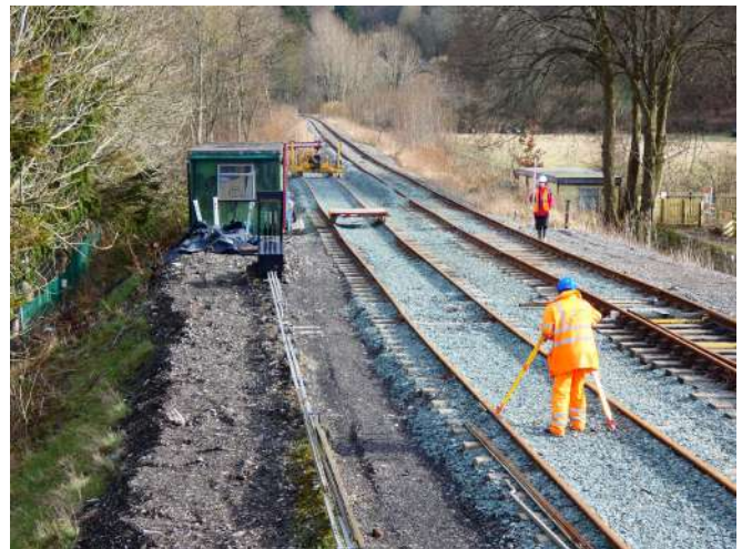
Peter Neve surveying rail top heights. The "umps and 'ollers" in the road are quite evident from this photo - plenty of tamping required here Photo: DT
