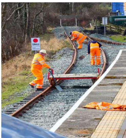
Work gang clearing ballast to make sleepers visible to the tamper operators Photo : DT
