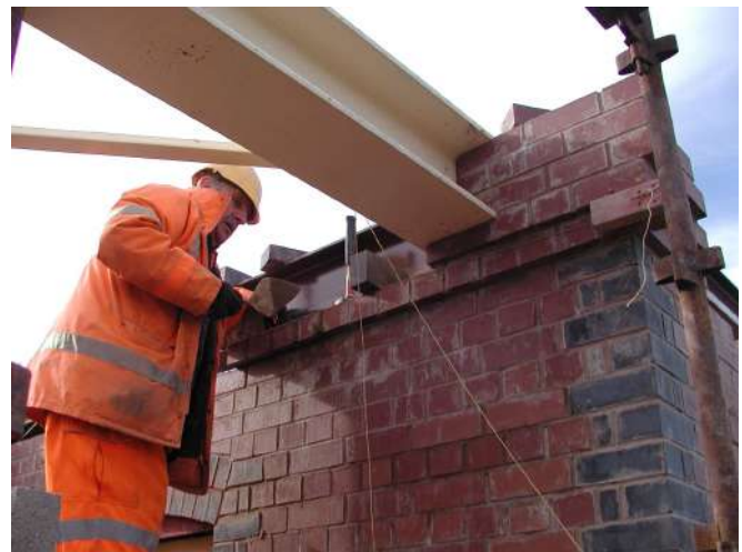
East Wall nearly complete. John Mason at work n the last couple courses Photo : PR
