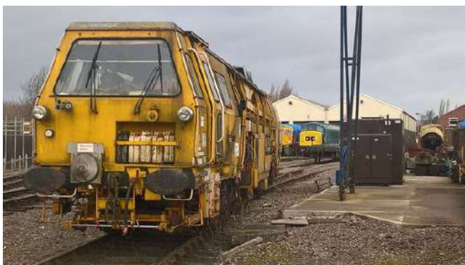
Bob Foster's Plasser Tamper at work on the GWSR during February Photo : B&R Track Services
