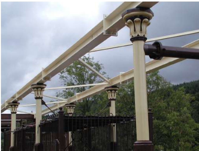
Cross bracing added to the carrier beams for added stability Photo : PR
