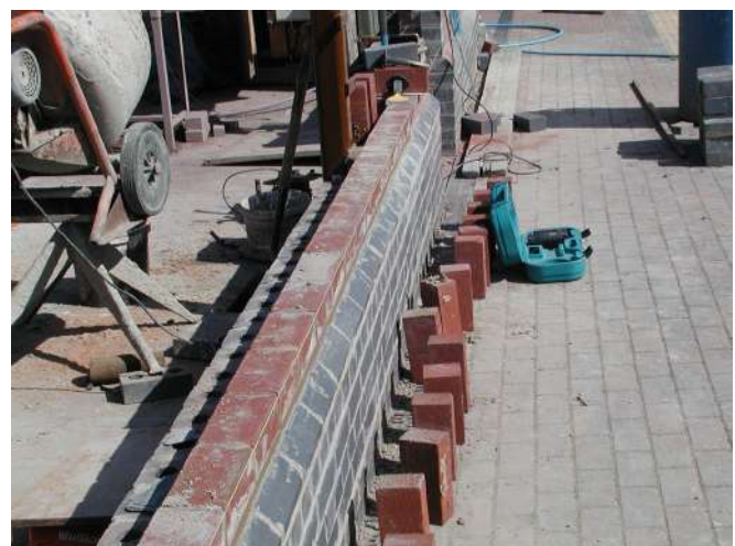
Red bricks added to the plinth course being bonded to the steel frame (top centre of photo) Photo : PR
