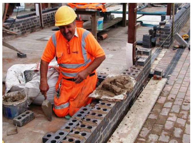
John Mason adding blue engineering bricks to the on-platform building Photo : PR
