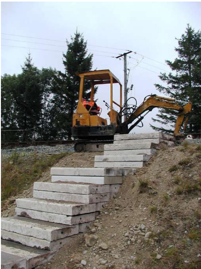
New East End steps up from the car park to rail level
