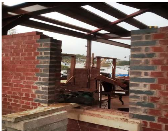
East wall height approaches the cross beam Photo: PR
