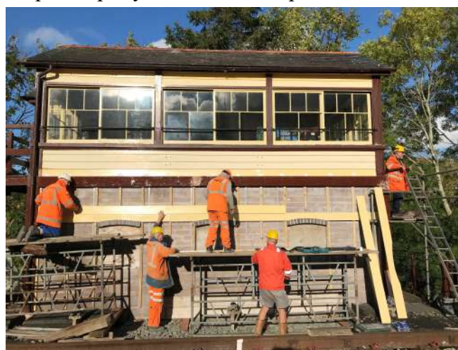
First pieces of cladding going on the front of the signal box
