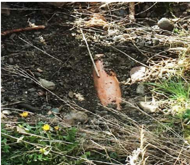
The sewer pipe awaiting permission to add "an arm's length" to connect to the main drain. Photo: PN
