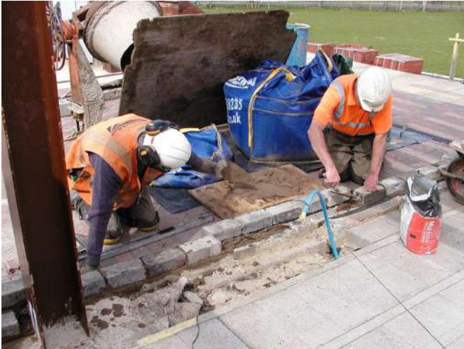
Joel Scott (L) and Peter Jump laying the first course of bricks on the station building Photo : PR
