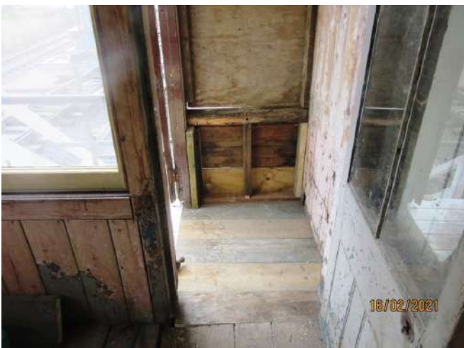
Porch floor boards complete offering a safe entrance to and from the stairs vv Photo: PM
