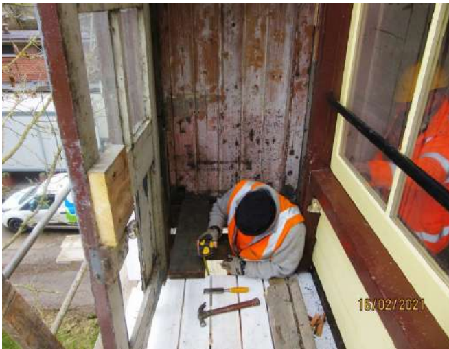
Peter Robson measures up for door clearance - standing on the scaffold below the porch! Photo: PM
