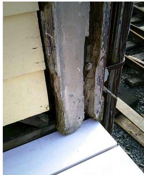
Poor condition of external corner post - compare new wood at top of stairs
