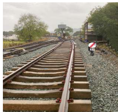
CN11 Shunt signal - UP siding to Platform 2 Source : HJP
