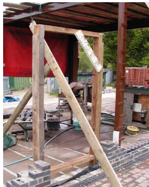
Door frame in place on the south side of the building Photo : PR
