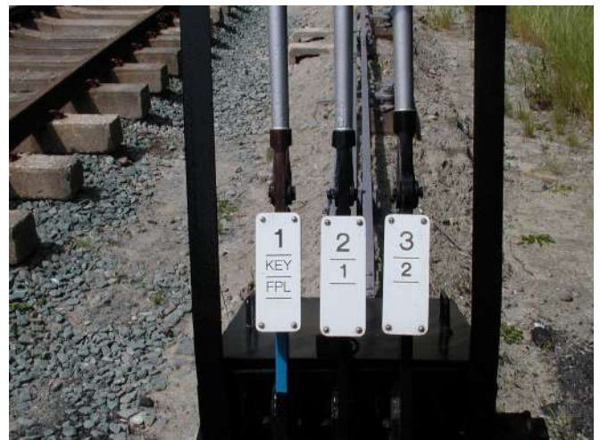
Operating levers for the East end ground frame - lever numbers and their action Photo : PR
