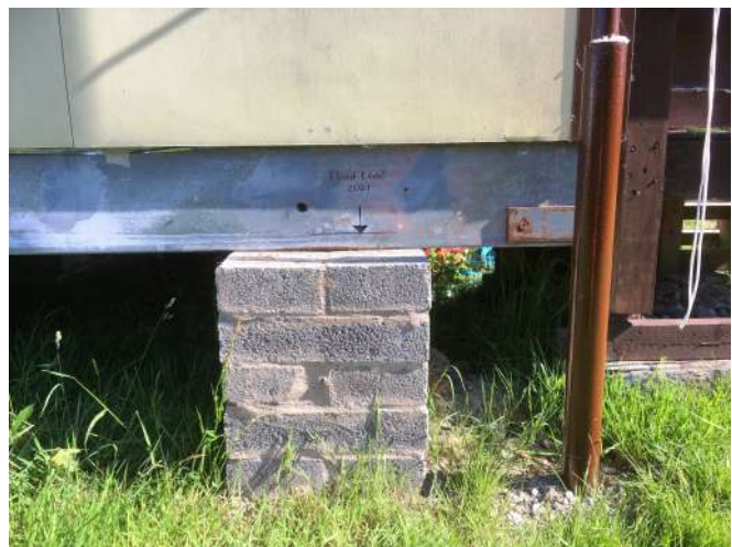
Flood marker - just below the ticket office floor Photo: PN
