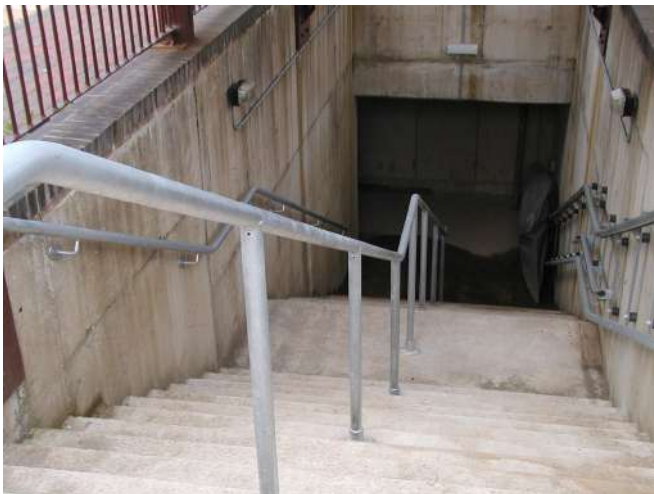
Stair rails installed on the access stairs to the island platform from the underpass Photo : PR
