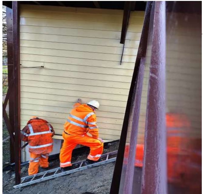
Last pieces of cladding being added. Note the steep angle of the embankment Photo : DT
