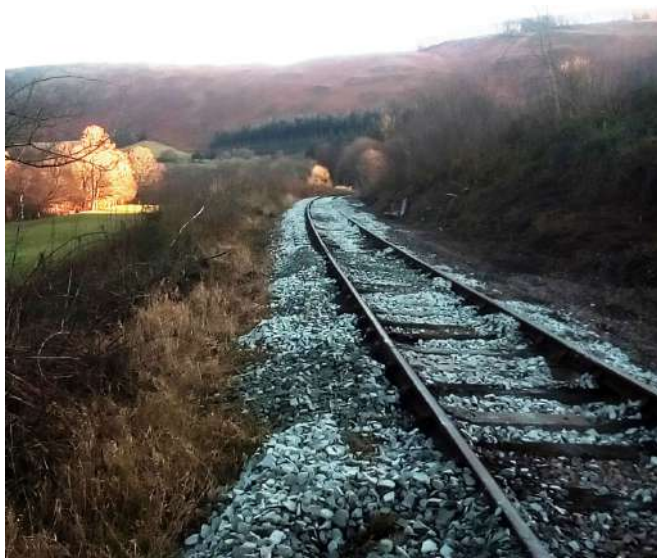
New Ballast and sleepers at Deeside catching the late afternoon sunshine Photo : PR
