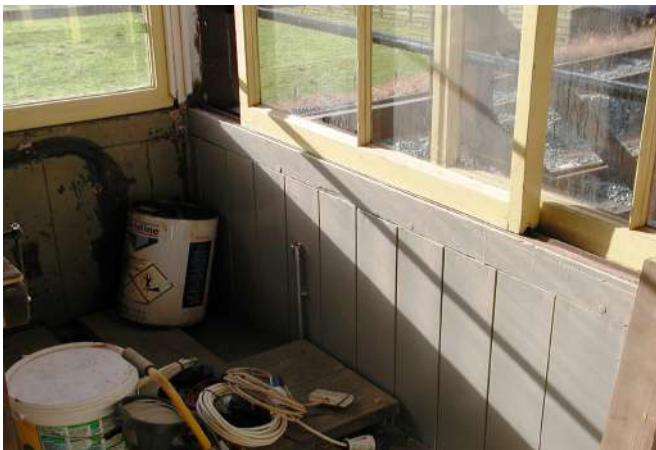
Undercoat on and electrical conduit coming up from the locking room Photo: PR
