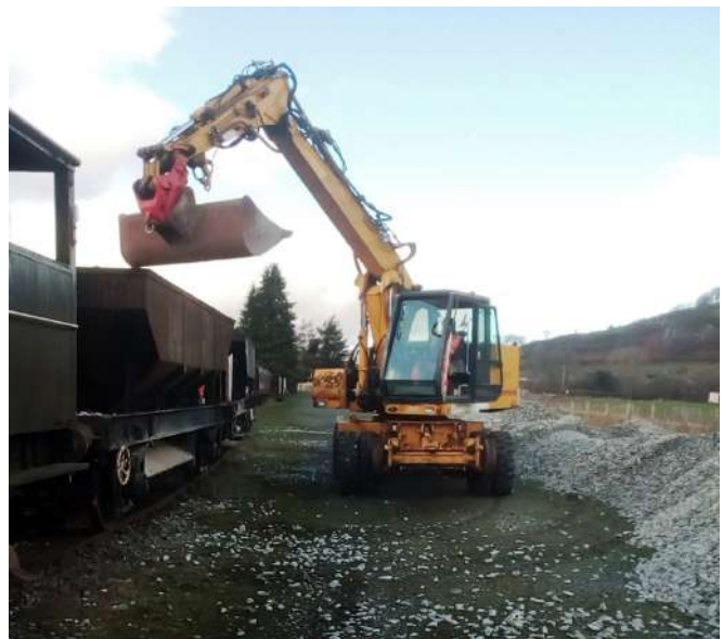
Rexquote-CASE busy loading ballast wagons in Carrog Yard ready to go east to Deeside Photo : PR
