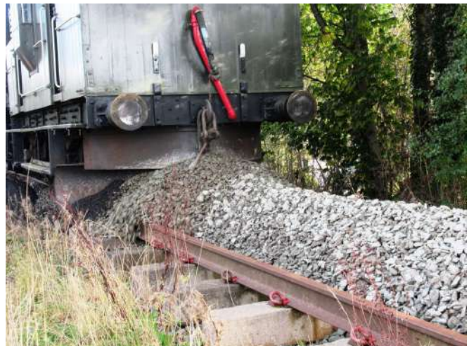
Ballast plough ready to push the stone to each side Photo : GJ
