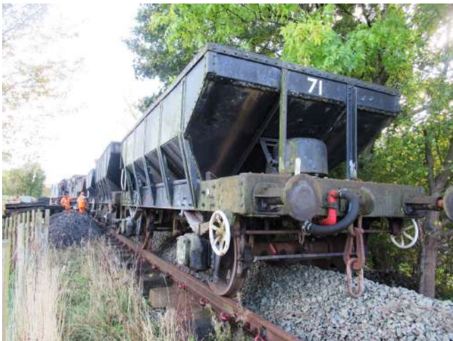
Ballast dropped in Green Lane Head shunt Photo : GJ
