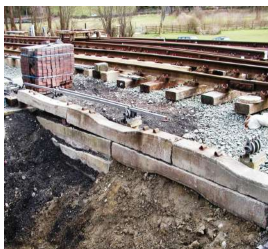
Concrete sleepers provide support for the track on top of the north batter Photo : PR
