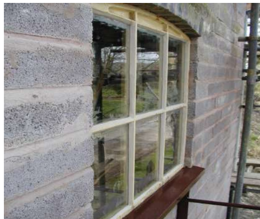
Glazed traditional arched frame windows at the back of the signal box Photo : PR
