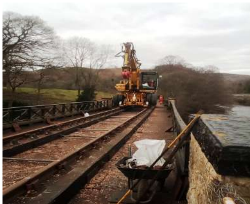
CASE/Rexquote RRV crosses the Dee on the newly relaid bridge timbers and rails Photo : PR
