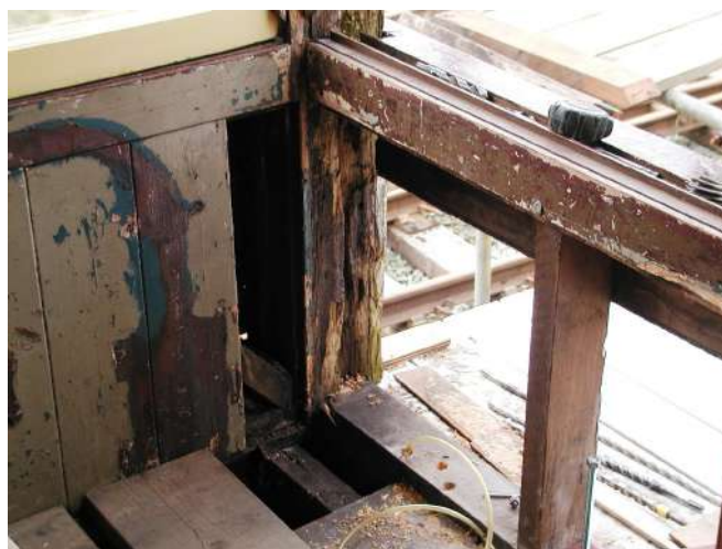
Wastage in the corner post by the staircase Photo : PR
