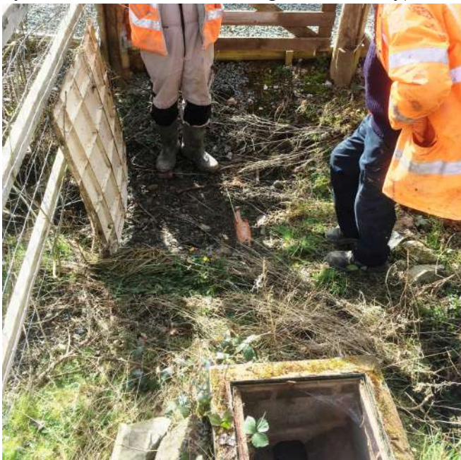
The railway's inspection chamber and the orange/brown adopted sewer pipe awaiting connection - a distance of barely half a metre! The gravel path visible in the background is where the connection chamber is on Betsi Cadwaladr's property
